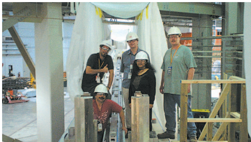
Figure 2. The POWGEN3 powder diffractometer team has completed installation of neutron guide. Photo credit: Luke Heroux/ORNL.
